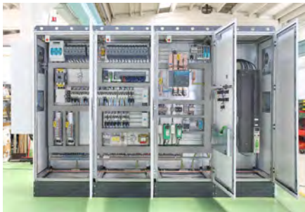
Nidec Drives supplied drive control technology to enhance FAE's recycling systems.
