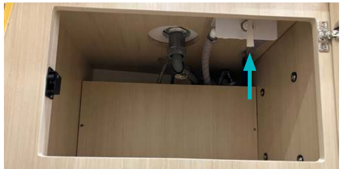
Shore water shutoff valve
