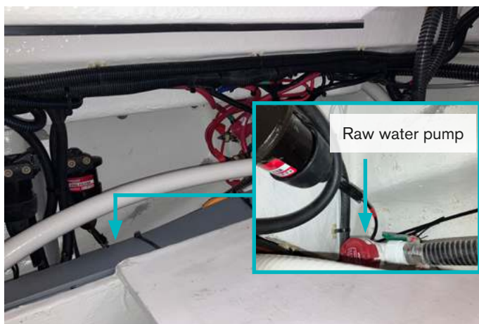
Port seacock and pump
