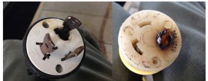
Examples of damaged shore power cords
