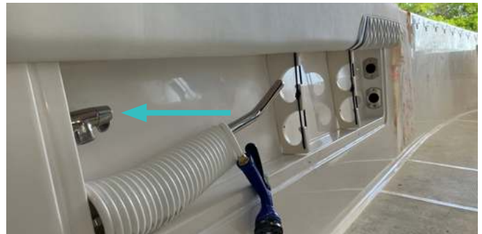
Port gunwale raw water washdown
