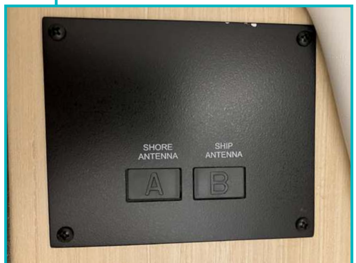
Coaxial splitter panel
