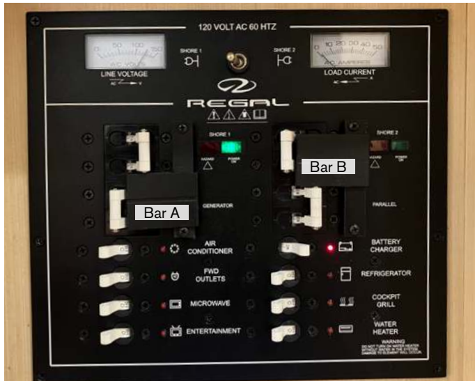
Main Distribution Panel (MDP)
