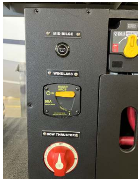
Bow thruster power switch
