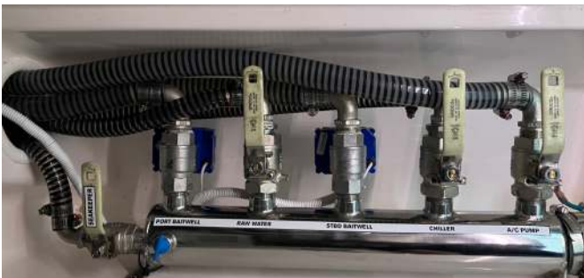
Raw water manifold
