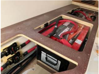
House and electronics batteries
