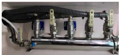
Raw water manifold
