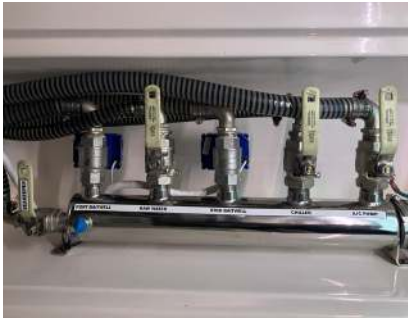
Raw water manifold
