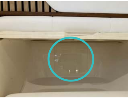
Water heater access panel
