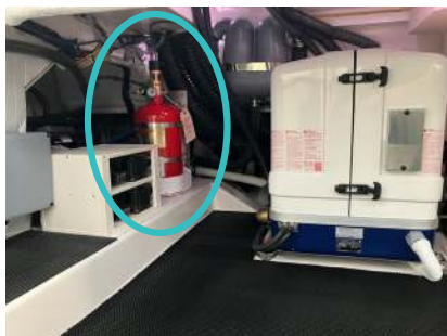
Fixed fire extinguisher
