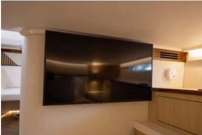
Mid-Berth CO/smoke detector
