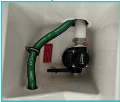
Overboard discharge location
