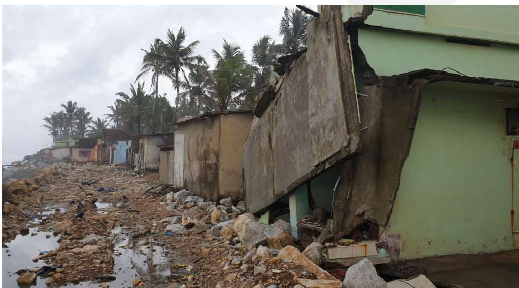
Fig.6 Houses damaged recently
