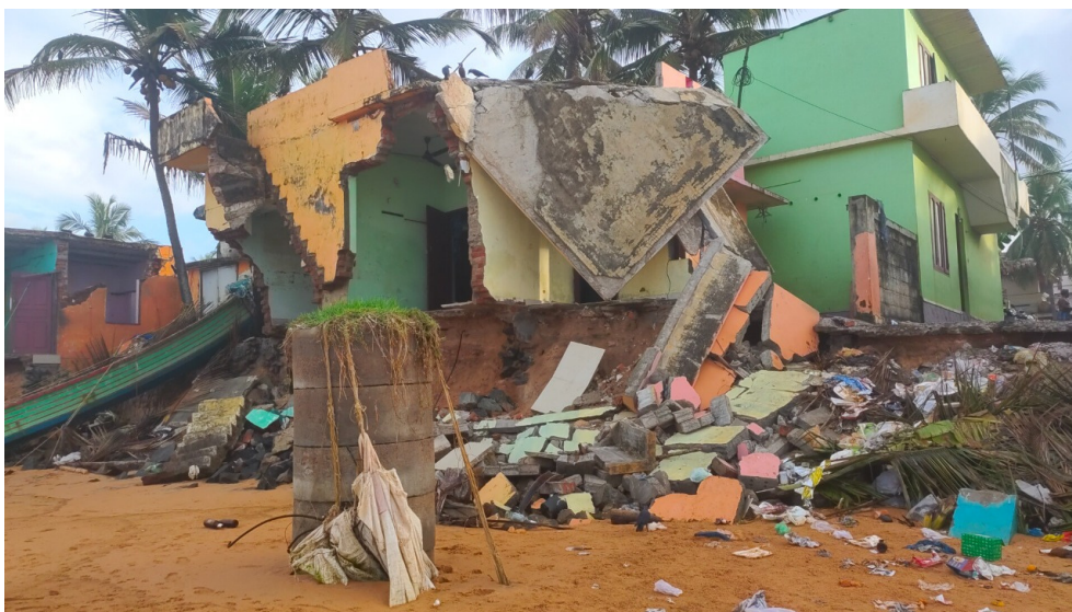
Highly Damaged Houses Near Valiyathura
