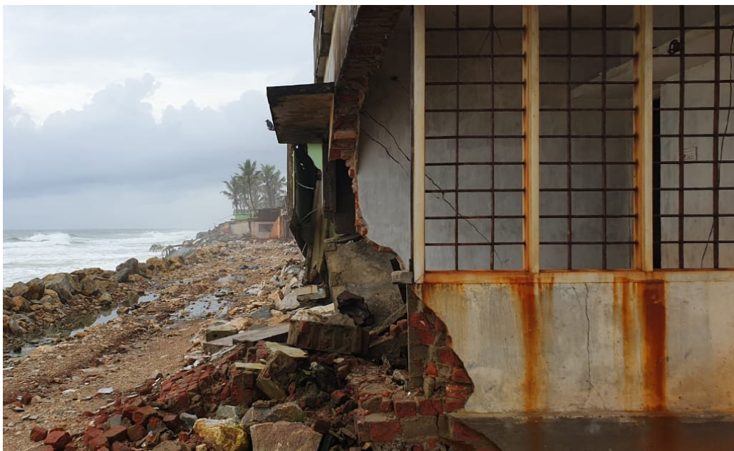
Fig.5 Houses damaged recently
