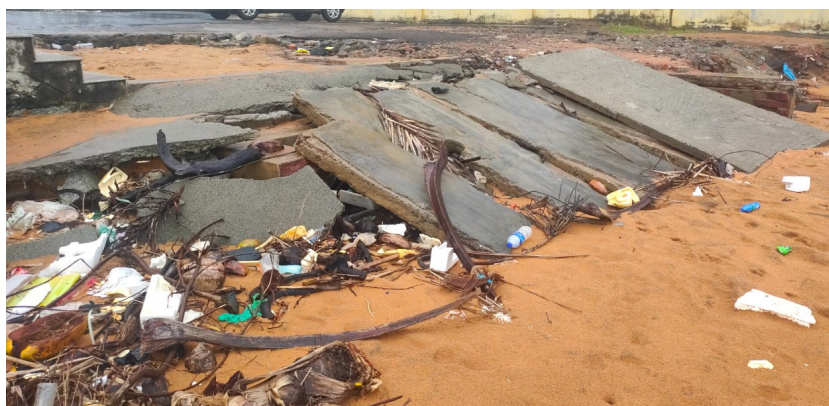
Fig.4 Steps damaged near Vettukadu Church
