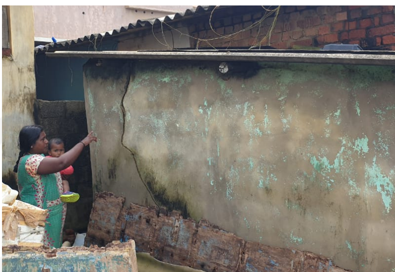
Fig.3 Houses damaged in Poonthura
