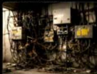
✗ Disorganized cable arrays
