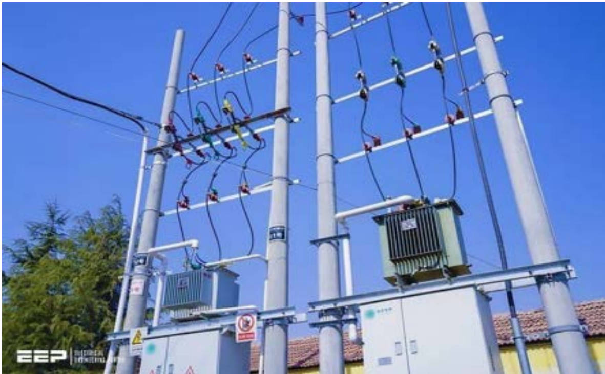
PROJECT- 500 KVA SUB-STATION GUWAHATI ASSAM CLIENT- ASSAM POWER DISTRIBUTION COMPANY (APDCL) Govt. Of Assam
