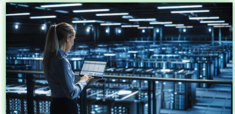
Micro Data Center and Server Room
