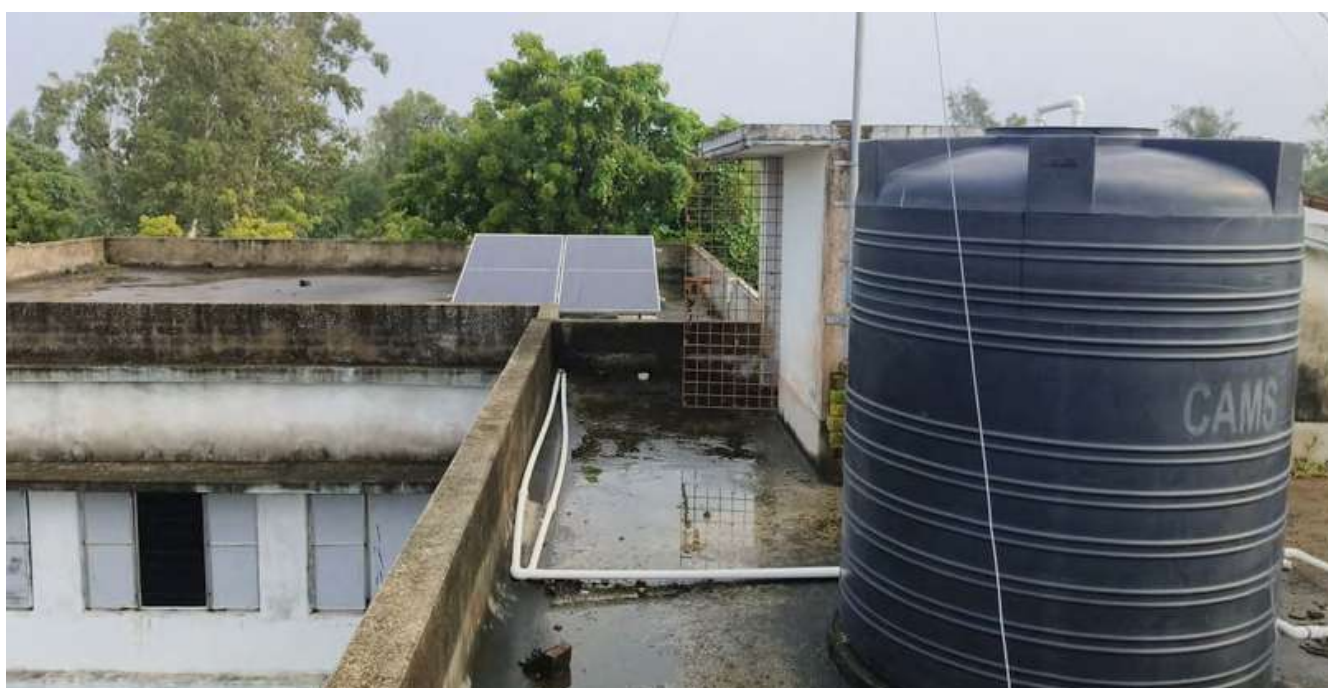
Photo 18: A solar powered storage tank at Raypara Pre-Primary School, Ghoramara Island
