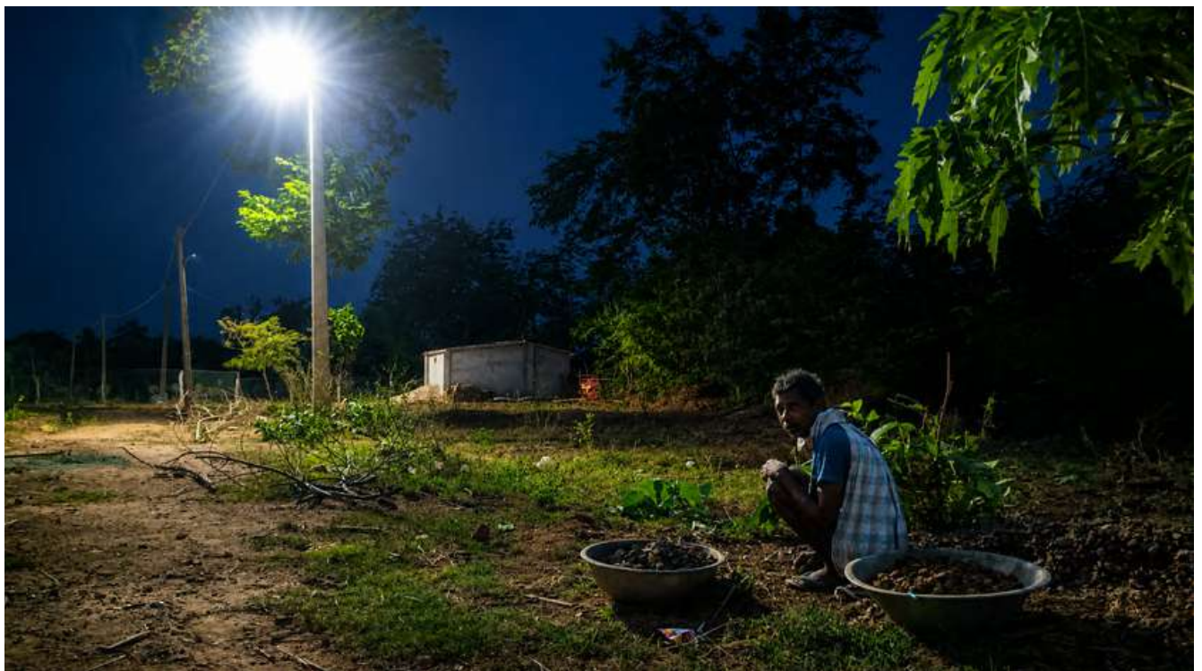
Photo 22: A solar street light in a forest fringe village of Betla National Park, Jharkhand
