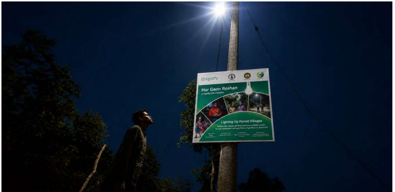
Photo 23: A solar street light in the forest fringe village of Palamu Tiger Reserve, Jharkhand
