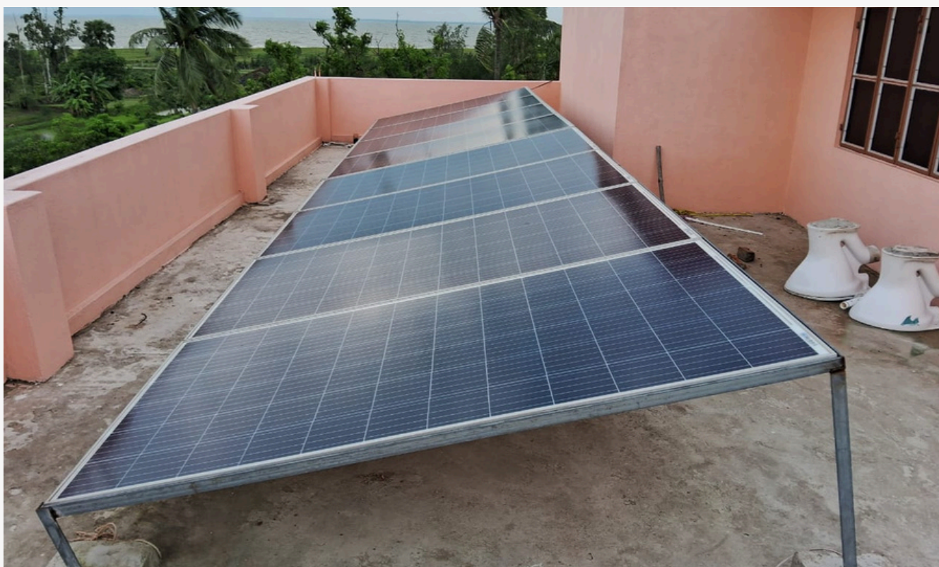
Photo: Rooftop solar array installed on the Multipurpose Cyclone Shelter, Raipara, Ghoramara
