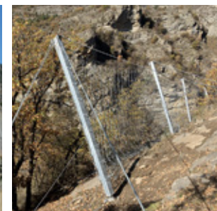
5 Dynamic Rockfall Barriers
