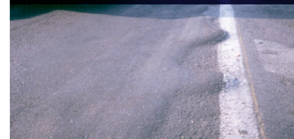
Rutting and shoving
