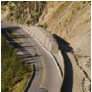
1 Rockfall and Landslide Embankments
