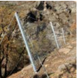
5 Dynamic Rockfall Barriers
