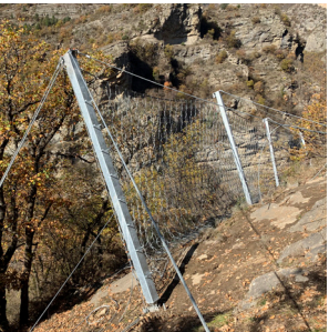
5 Dynamic Rockfall Barriers
