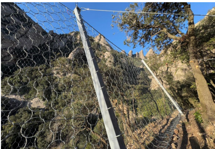
RB3000 barrier seen from the mountain side
