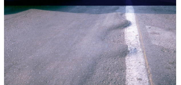
Rutting and shoving
