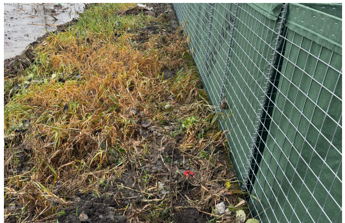
After: White River Flood Protection Barriers
