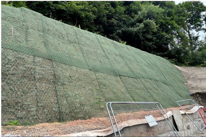
MacMat erosion control layer
