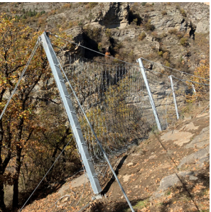
5 Dynamic Rockfall Barriers
