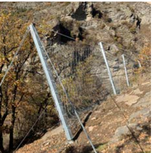
5 Dynamic Rockfall Barriers
