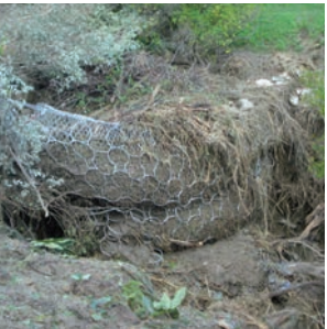
4 Debris Flow & Shallow Landslides
