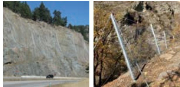
2 Mesh Systems - Simple Drapery 5 Dynamic Rockfall Barriers
