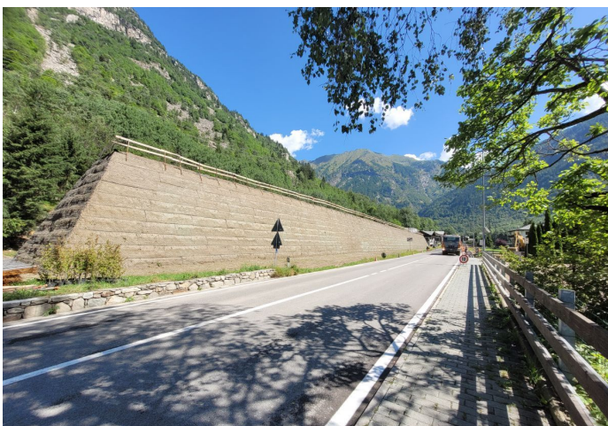
Rockfall barrier detected in Terramesh Verde protecting
