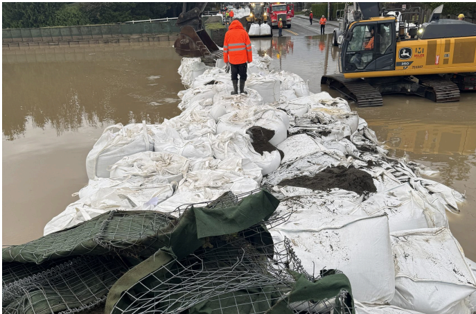
Before: Previous Breached Flood Barrier System
