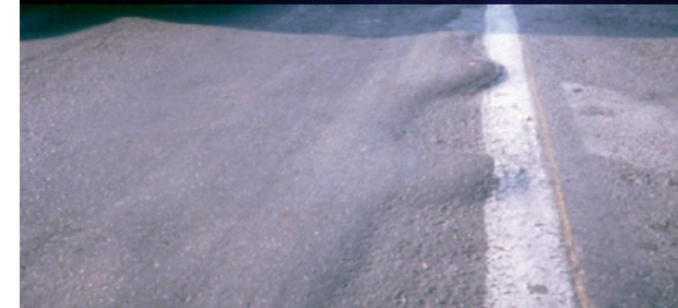
Rutting and shoving
