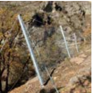
5 Dynamic Rockfall Barriers
