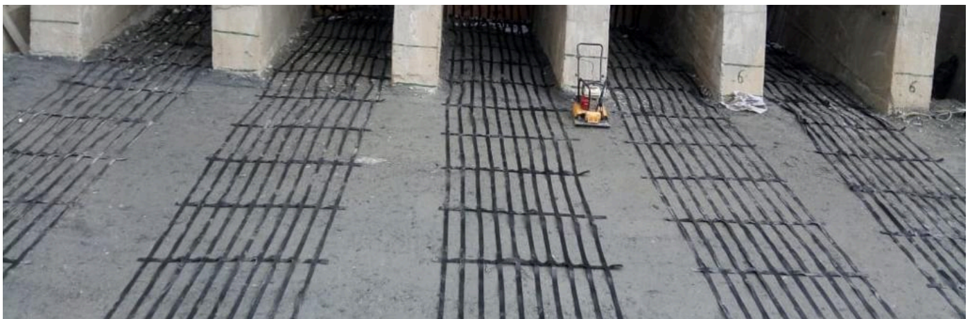
Use of Plate compactor near to structure
