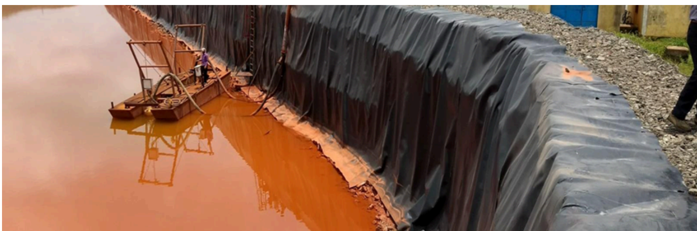
PHOTOGRAPH SHOWING THE COMPLETE INSTALLATION ON THE BOUNDARY LOCATION OF THE POND
