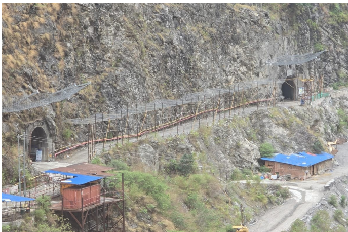
Fig-7 Rockfall Barrier above Desander basin upstream and
