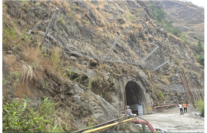
Fig-6 Rockfall Barrier above Desander basin downstream
