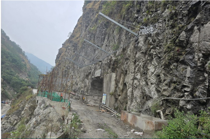
Fig-5 Rockfall Barrier above Desander basin upstream access
