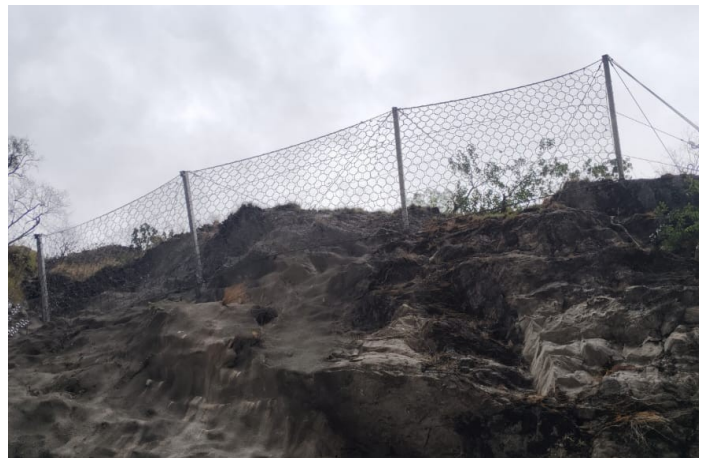
Fig-8 Rockfall Barrier above power intake access portal
